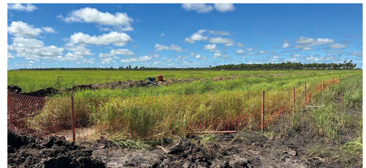
玻利维亚项目生态保护管线施工防止动物坠落 Ecological protection measures implemented for the project in Bolivia to prevent animals from falling into the excavated areas
